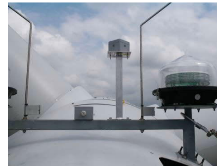
Figure 2. Sensor mounted to the top of a wind turbine nacelle.
